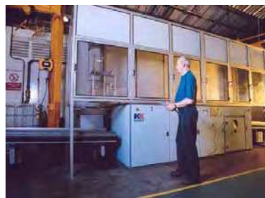
Figure 16 - Solvent Vapor Recovery
