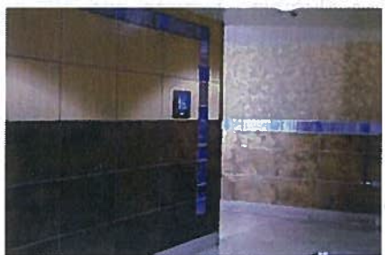
EXAMPLE OF GLASS ACCENT TILE BANDS AT SEA-TAC AIRPORT'S BAGGAGE CLAIM RESTROOM (TILE CREATOR: NORMANCOURTNEY)
