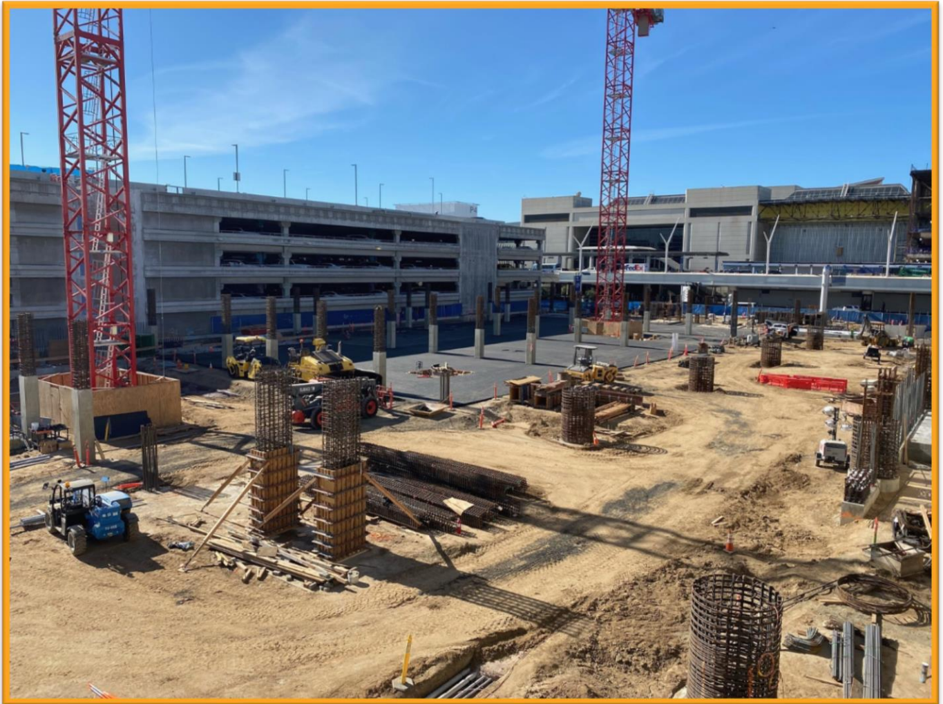
Automated People Mover paving of Ground Level at future West Station site between Parking Structures 3 & 4
