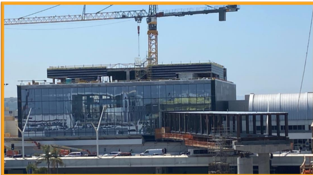
Current progress on Terminal 4.5 (Curtain wall complete, APM pedestrian bridge under construction)
